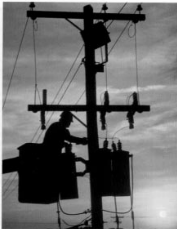
1. Work location should be assessed for available fault current and fault clearing time to determine how much protection is it needed
