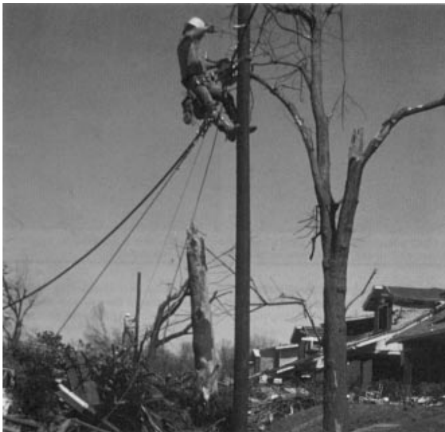
6. Under storm restoration conditions a good rainsuit, with suitable undergarments, may provide protection from possible arcs, and from the weather
